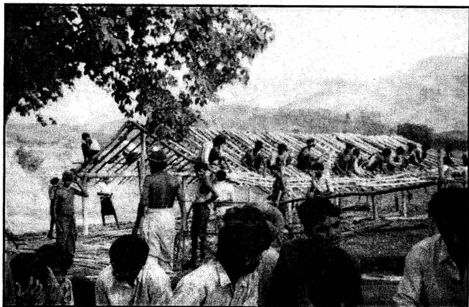
Indian villagers building new housing for the many families moving into the area being submerged
